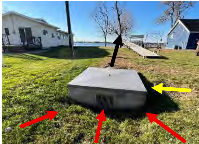
Stormwater catch basin – black arrow shows water leaving by underground pipe to outlet. Yellow arrow shows water from underground pipe from driveway culvert flowing into catch basin.
