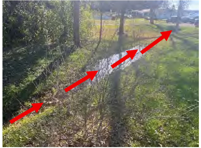
Water from County Rd 47 culvert heading towards driveway culvert
